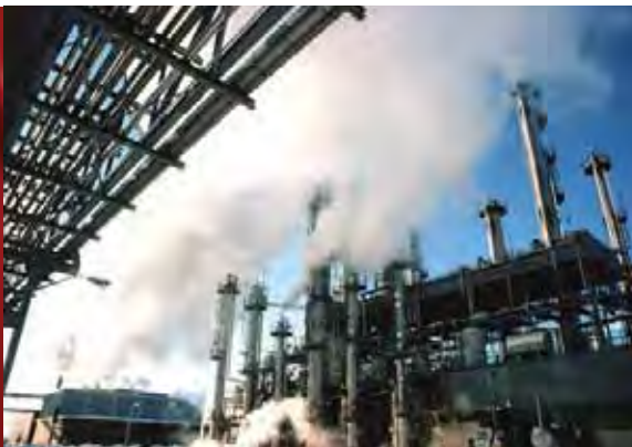
Instrumentation and Automated Pneumatic Controls
